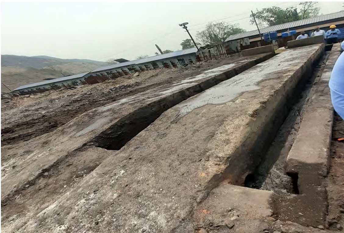
Washing platform in Godhur opencast coal mine
