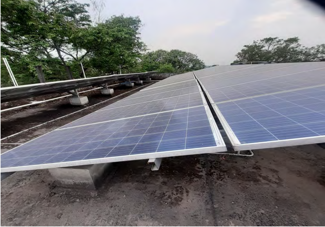
Rooftop in solar panels
